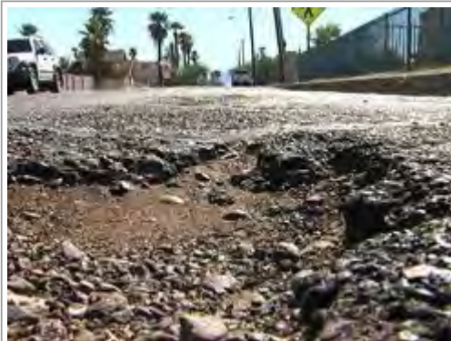
Pothole at 14th St. & Garfield in Phoenix (Tim Vetscher)
